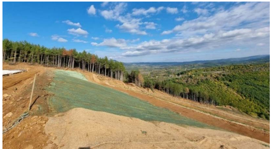
Grassing through the method of hydroseeding is an effective way to establish vegetation on large areas of land
