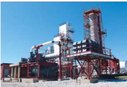
New oxygen plant at Tsumeb smelter.
